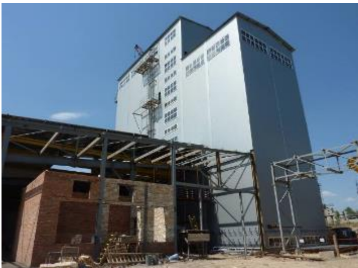
The sheathed Batch house and Big-bag storehouse
