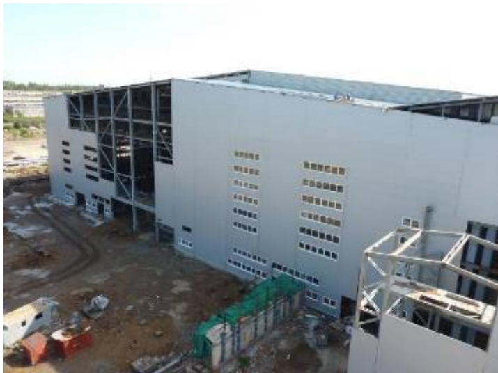
Production monoblock (Metallurgical hall)
