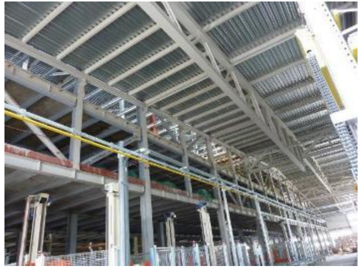
Production monoblock (Metallurgical hall)
